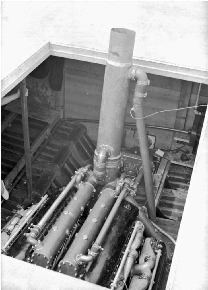
Figure 18 ORCA engine room. Note arrangement of the water cooled exhausts, the short extension shafts, “AEC” logo on the valve covers and the streamlined intake manifolds installed when the engines were modernized.
